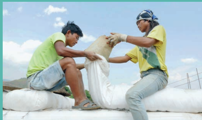
Men add soil to an Earthbag, made of polypropylene fabric that is estimated by the U.S. Highway Safety Administration to have a tensile strength greater than steel.
